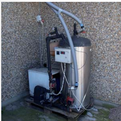
7 kW cooling system for floor cooling.
