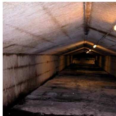
Even though the duct of plywood is insulated, fungi still form on the boards.
