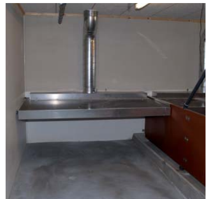
Supplemental air intake through nozzles under the cover.
