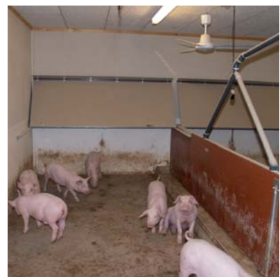
Ceiling fan installed above a finisher pen.
