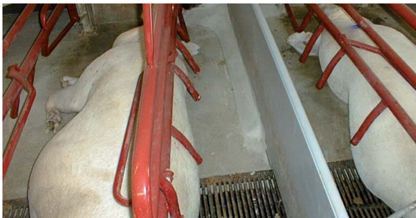
It is still recommended to have an area filled with concrete between the pen side and the floor in order to reduce the risk of mess on the solid floor.
