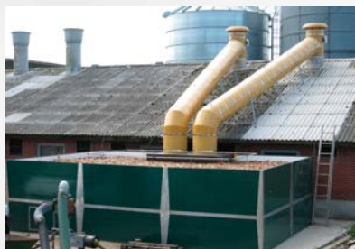
The BIOREX-Hartmann biofilter established by a finisher facility.
