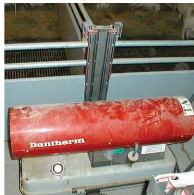
In a facility of approx. 200 m 2 , approx. 75 l oil are typically required to dry up the facility.
