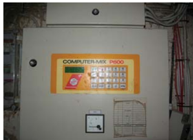
Check the consumption of ingredients and the mixing accuracy in your on-farm mixing system.
