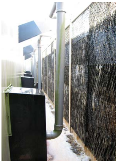
ScanAirclean's central purifier from the Dutch company INNO+.
