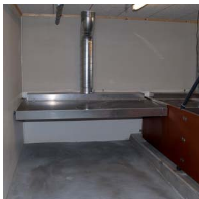
Supplerende luftindtag via dyser under overdækning.
